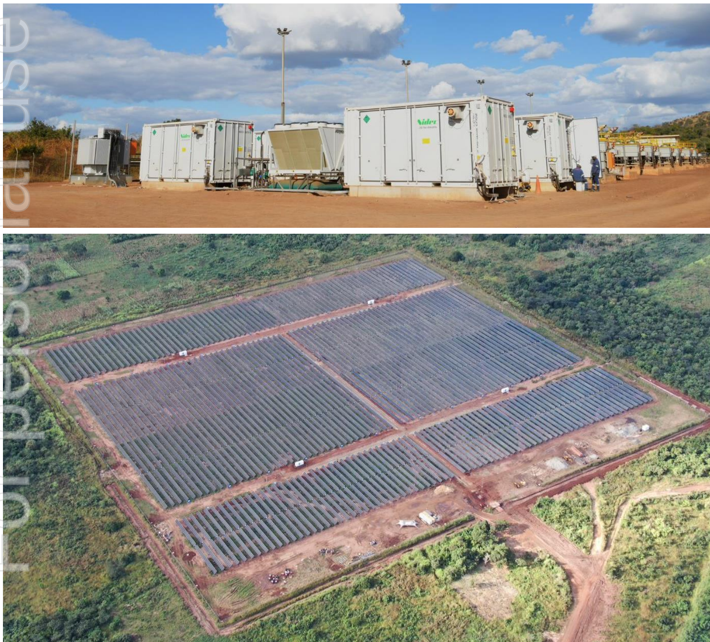
Figure 1: Balama Solar & Battery System.
