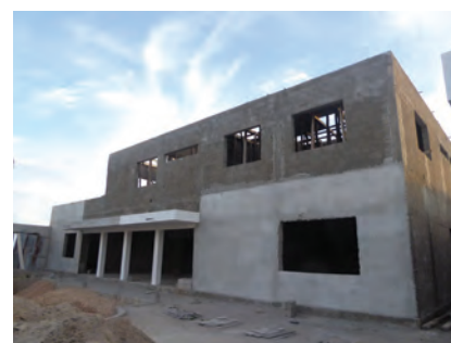
167_Unpermitted construction_site B.JPG
