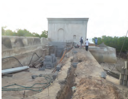
160_Unpermitted construction_site A.JPG
