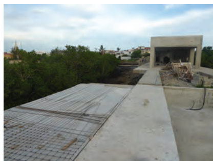
162_Unpermitted construction_site A.JPG
