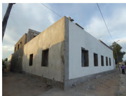
165_Unpermitted construction_site B.JPG
