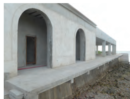
161_Unpermitted construction_site A.JPG
