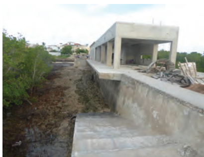
163_Unpermitted construction_site A.JPG
