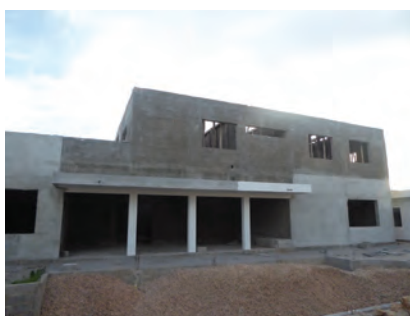
166_Unpermitted construction_site B.JPG
