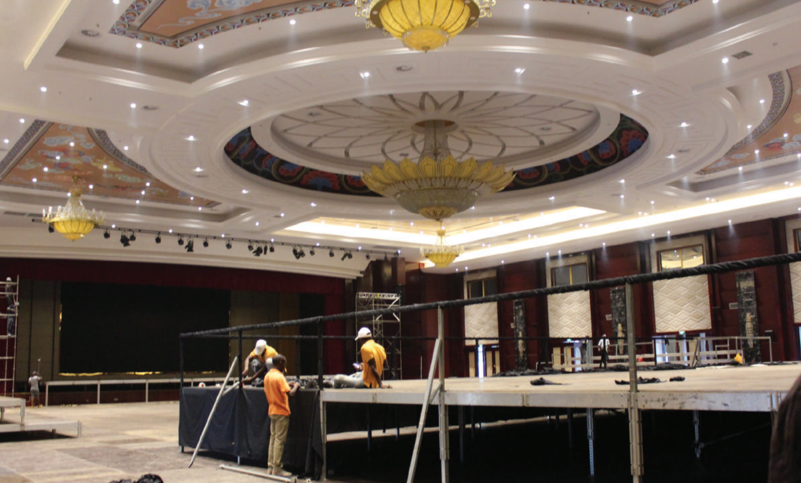
Renovations at the Polana Hotel in Maputo, meeting place of the Mozambican elite and international visitors (photo Estacio Valoi)
